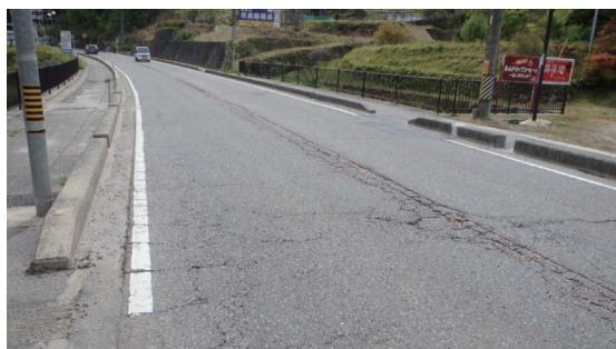
Damaged road pavement
