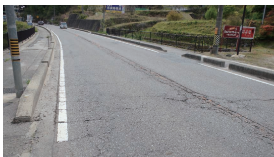
Damaged road pavement
