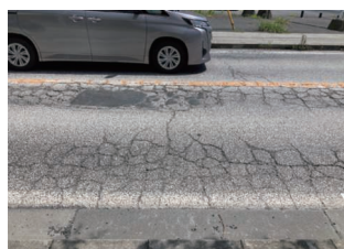
Cracks in pavement
